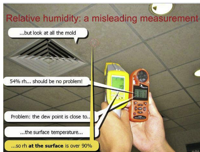
Figure 9. Temperature and humidity are not uniformly distributed throughout a house. The ceiling near the air conditioning supply vent has been chilled by the cold air to a temperature low enough to condense moisture and support dust mite and mold growth. Other locations inside a typical house may have similar micro-environments with excess or accumulated moisture.
